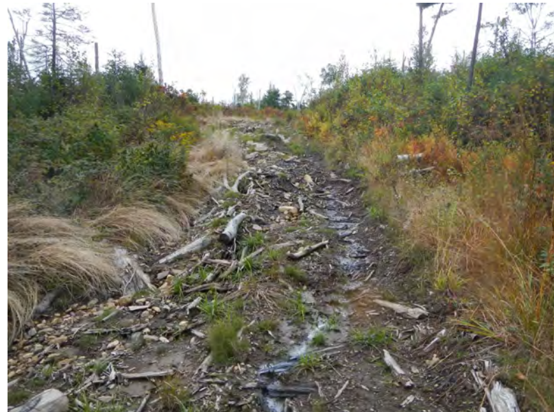
Figure 23: Severe Erosion- The primary access trail into the property from Dyke Road-Jim Noyes Hill Road has significant erosion problems.
