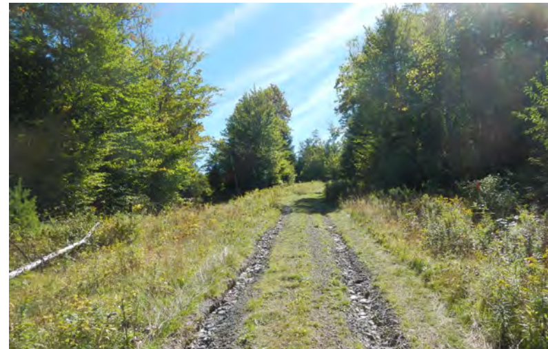
Figure 22: Erosion- Part of the Merrill Mountain Road access and private access roads that serve the property are starting to erode.
